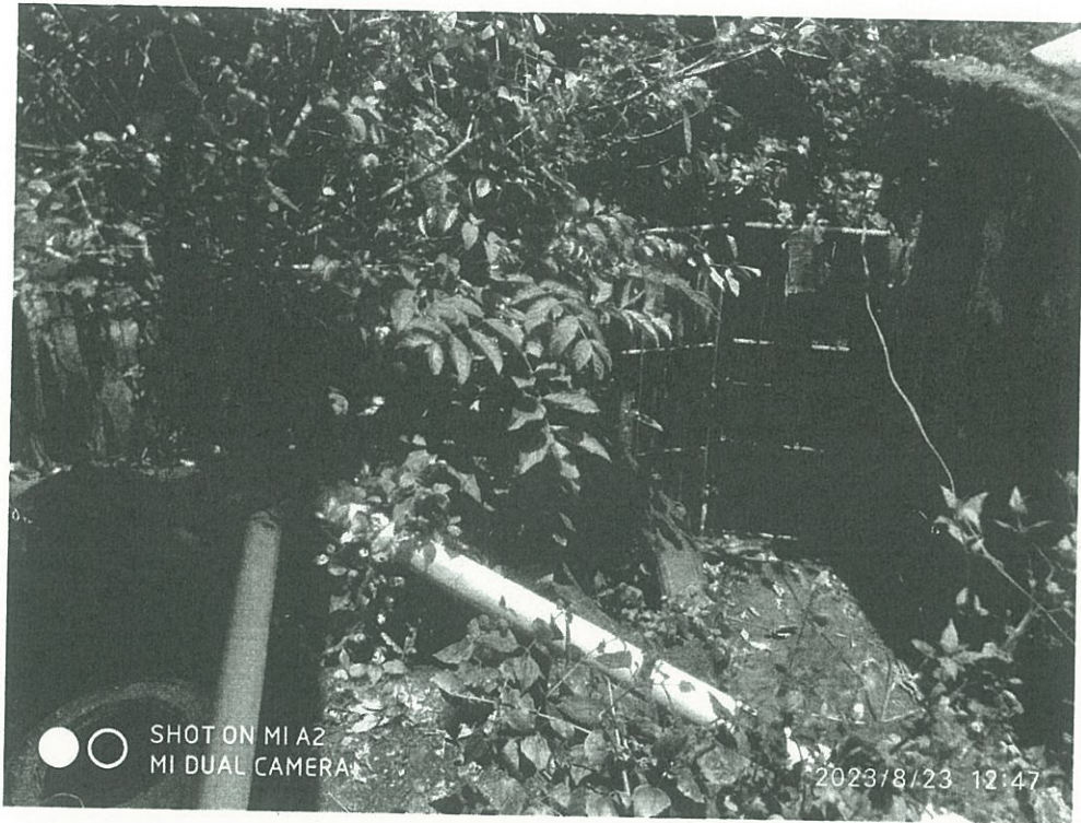
EASTERN SIDE BOUNDARY WALL WITH APPROX. 1.2m WIDE METAL GATE OPENING FROM SOUTH-EAST SIDE
